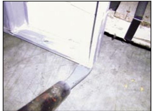
Or, place the slip bar under the gusseted corner of the form.
